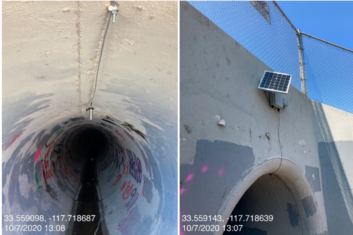
Figure 6. Example of outfall installation with smart gateway, solar panel, regulator and battery enclosure, and downward looking ultrasonic sensor.
