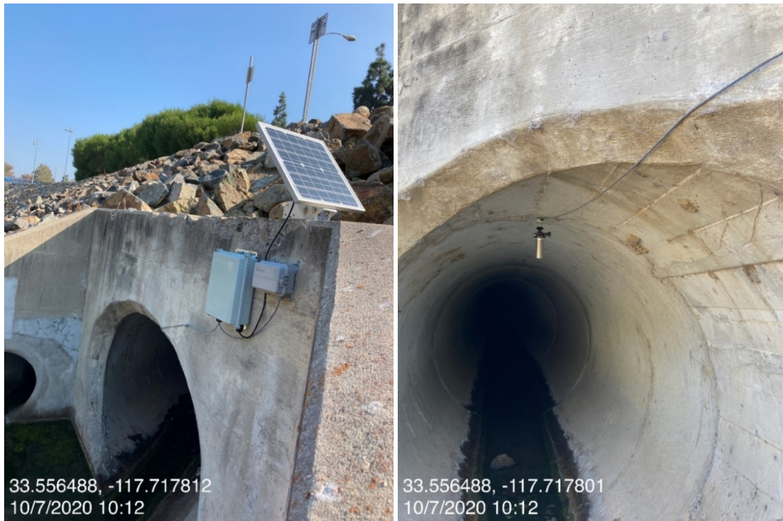
Figure 7. Example of outfall installation with smart gateway, solar panel, regulator and battery enclosure, and downward looking ultrasonic sensor.
